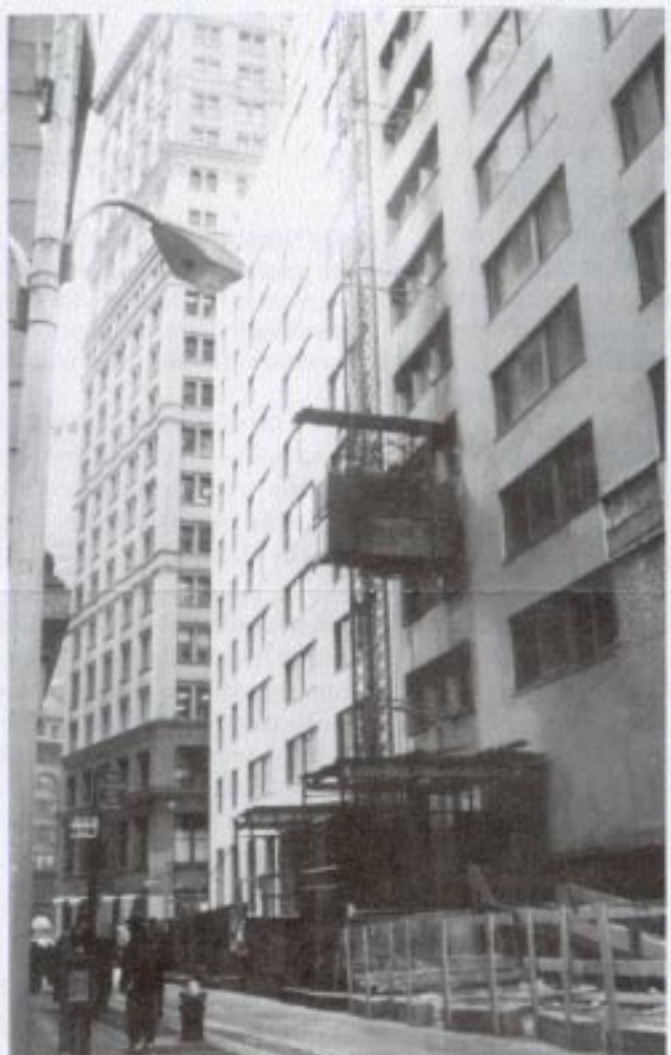
Former Atlantic Mutual Building at 45 Wall Street is undergoing a transformation to residential use, just one of dozens of projects that are revitalizing lower Manhattan.
