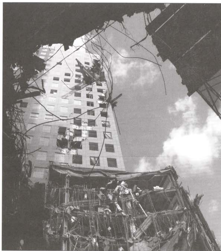
A beautiful, clear sky contrasts with massive damage suffered at New York's World Financial Center on 9/11. Photo was taken from inside the Winter Garden.
